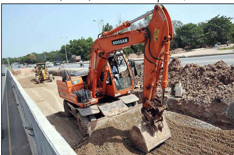
ISLAMABAD: Heavy machinery being used for expansion work of Club Road during development work in Federal Capital.
