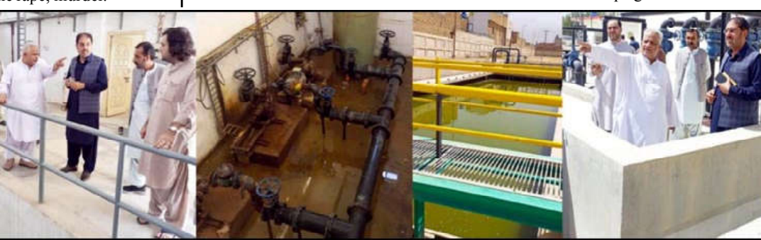
QUETTA: Caretaker Provincial Minister for PHE & Population Welfare Sardar Ejaz Ahmed Khan Jaffar inspecting water treatment plant and booster pump at Sabzal road.
