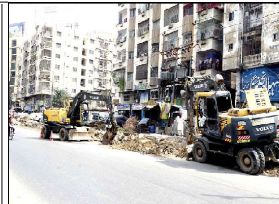
KARACHI: Construction works of new development projects for extending road is underway under the supervision of local government department, as slow pace of construction work is creating problems for commuters due to traffic jam and they demand to concerned department to complete work as soon as possible, located on Shahrah-e-Faisal road in Karachi.
