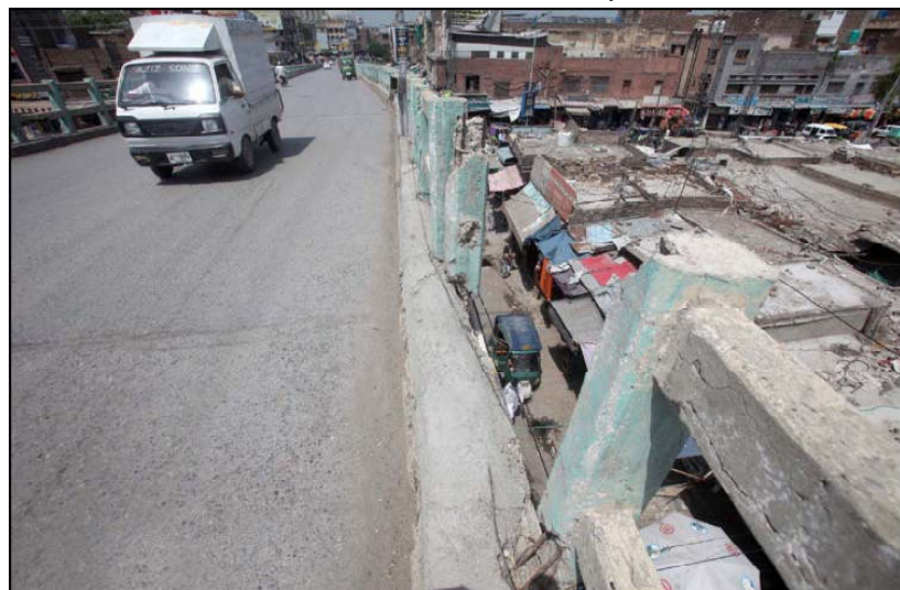
PESHAWAR: Safety wall of Faqirabad Bridge seen broken that may cause any accident and also inviting authorities to draw their attention towards issue, in Peshawar.
