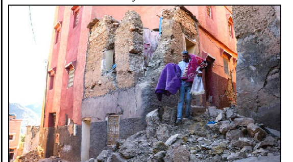
A man carries belongings out of his damaged house, in the aftermath of a deadly earthquake in Moulay Brahim, Morocco
