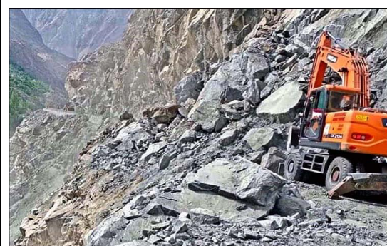
GILGIT: FWO workers busy in clearing block area of Juglote-Skardu road after land sliding during rain in city.
