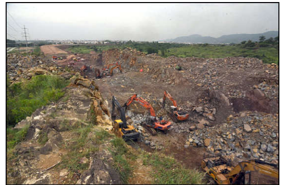
ISLAMABAD: A view of the heavy machinery on the sight of the Khayaban-e-Margalla as the construction work of next part is being completing very efficiently in Federal Capital.
