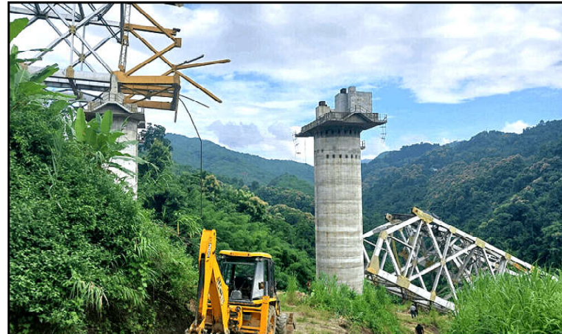
Rescue workers conduct a search operation at the site of an accident where an under-construction railway bridge collapsed in Sairang town of the Aizawl district in India's eastern state of Mizoram.
