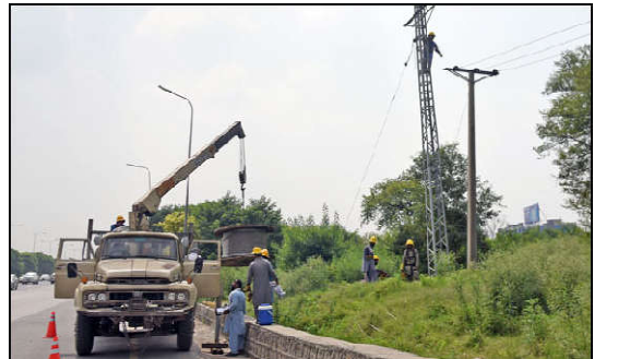
ISLAMABAD: WAPDA workers are busy in installing electric wires on poles along the Express Way during high temperature in Federal Capital.
