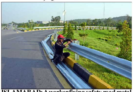
ISLAMABAD: A worker fixing safety road metal beam for traffic at 7th avenue bridge in Federal Capital.
