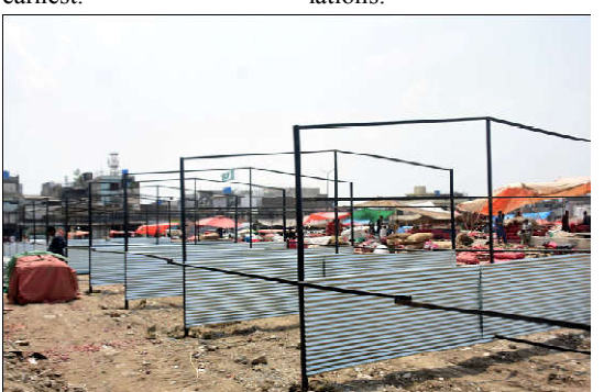
ISLAMABAD: A view of the newly made cabins at Fruit and Vegetables Market as the vendors are unhappy due to its quality and the size of cabins as the Anti encroachments cell demolished their cottages to install such new one, on monthly rental basis in Federal Capital.
