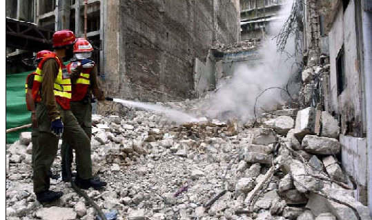
KARACHI: View of site after a fire broken out incident as the fire brigade officials are busy in extinguishing fire and rescue operation, located on LI Chundrigar road in Karachi.
