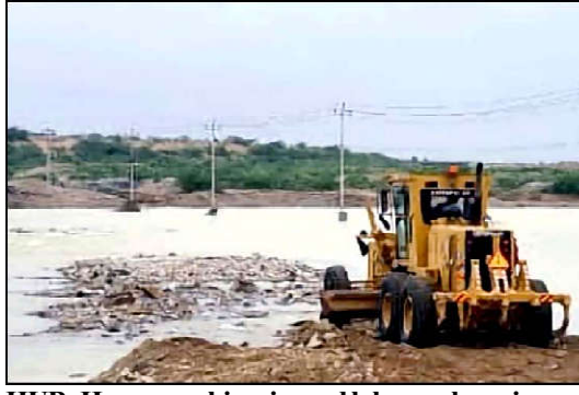
HUB: Heavy machineries and laborers busy in construction work of Causeway crossing road that was completely destroyed after flood flowed in Hub River during recent heavy downpour of monsoon, under the supervision NHA, located on Hub River road in Hub.
