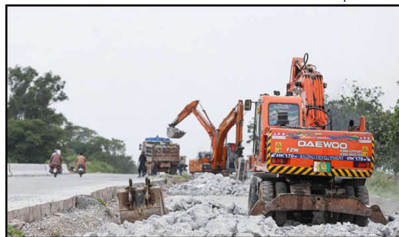
ISLAMABAD: Heavy machinery is being used to expand lanes for smooth traffic on Islamabad Expressway.
