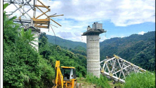
Rescue workers conduct a search operation at the site of an accident where an under-construction railway bridge collapsed in Sairang town of the Aizwal district in India's eastern state of Mizoram.
