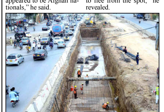
KARACHI: A view of ongoing construction work of Red Line Bus Service named as (Peoples Bus Service) at University Road in Provincial Capital.
