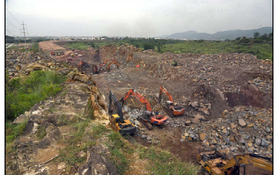
ISLAMABAD: A view of the heavy machinery on the sight of the Khayaban-e-Margalla as the construction work of next part is being completed very efficiently in Federal Capital.
