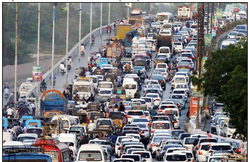
KARACHI: A large numbers of vehicles stuck in traffic jam due to construction and repairing work of Natha Khan Bridge located on Shahrah-e-Faisal in Karachi.
