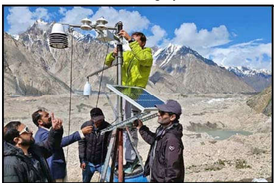
GILGIT: In the collaboration of EPI Gilgit-Baltistan, KTU, UOB, and University of Maitlaan EvK2CNR successfully installed the Automate Weather Station in Askoli, Urdas and Candolia.
