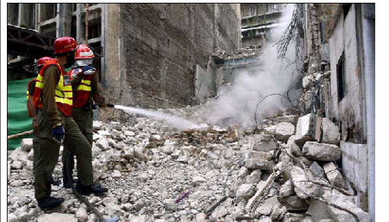
KARACHI: View of site after a fire broken out incident as the fire brigade officials are busy in extinguishing fire and rescue operation, located on LI Chundrigar road in Karachi.
