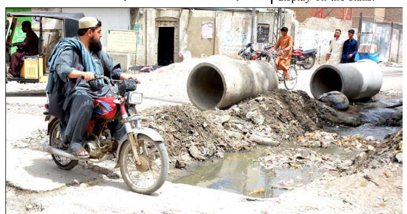
QUETTA: A view of sewerage water accumulated on Sirki Road Gawalmandi Chowk which creating problems for motorists need attention of concerned authorities.
