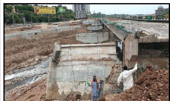
RAWALPINDI: Labourers busy in construction work underway on the collapsed bridge at Swan near High Court.
