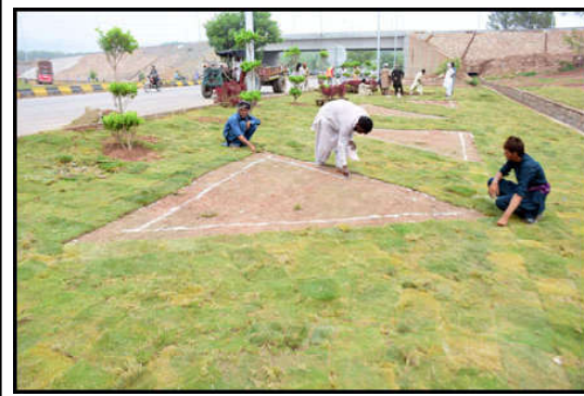
ISLAMABAD: Workers of Capital Development Authority (CDA) are busy in giving final touch to the newly constructed Bara Kaho Interchange to meet the dead line for inaugurating by PM in Federal Capital.
