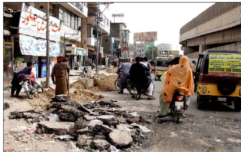
QUETTA: Laborers are busy in digging works while commuters are facing difficulties in transportation due to development works, as slow pace of construction work is creating problems for residents and they demand to concerned department to complete work as soon as possible, in Quetta
