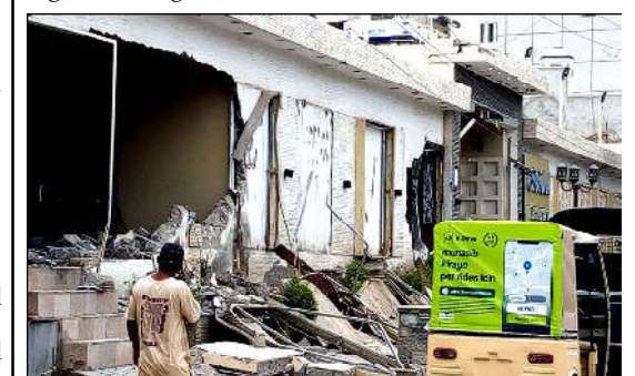
KARACHI: Anticreachment authorities demolishing illegal marriage halls constructed on residential land, during anti encroachment campaign under the supervision of local government departments located on Malir Model Colony area
