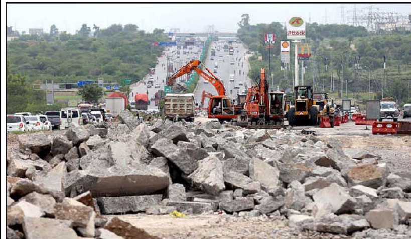
ISLAMABAD: Heavy machinery being used to expand Islamabad Expressway during development in Federal Capital.
