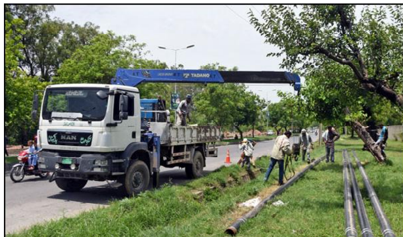
ISLAMABAD: Workers of local administration are installing gas pipe lines along the Park road in Federal Capital.
