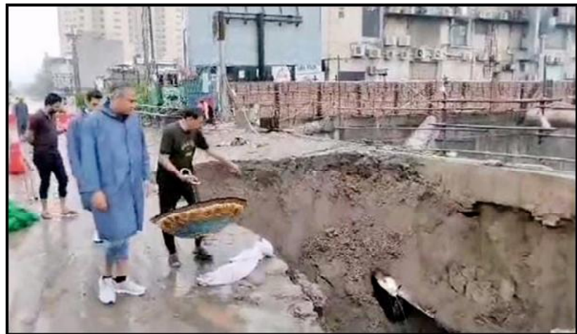
LAHORE: Caretaker Chief Minister Punjab Mohsin Naqvi paying a visit to different areas of Lahore in rain, issues directions to the administration and WASA officials for speedy water drainage.
