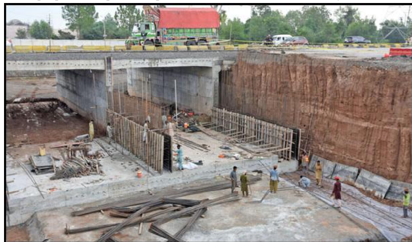
ISLAMABAD: Laborers are busy in their work during the construction of Margala Under pass. A street vendor is roasting the Corns in traditional mud oven on his handcart along the Murree Road in City.
