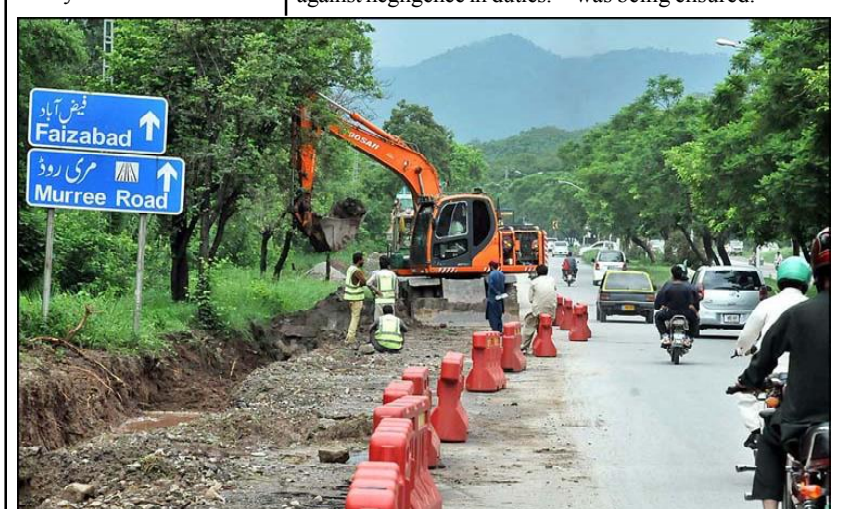
ISLAMABAD: During the expansion work of Club Road, heavy machinery is being utilized to carry out the construction and development tasks.
