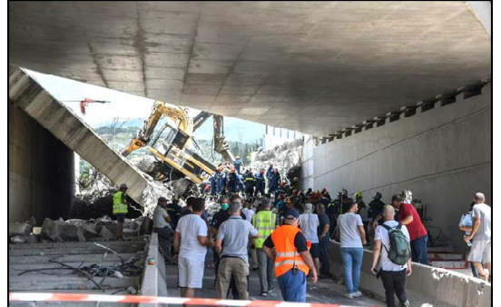
People are seen at the site of a bridge that collapsed in Patras, Greece.
