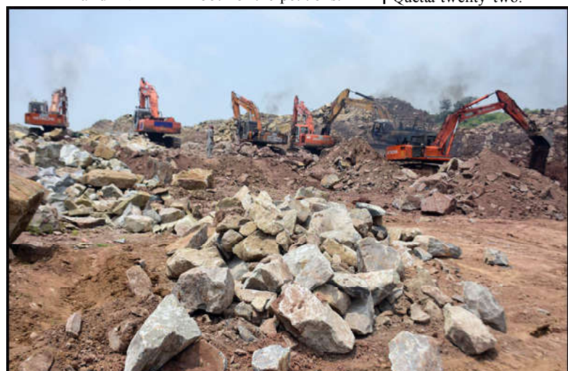
ISLAMABAD: Workers are busy in their work at the site of Khayaban-e-Margalla road, as the construction work is keep going gradually, in Federal Capital.
