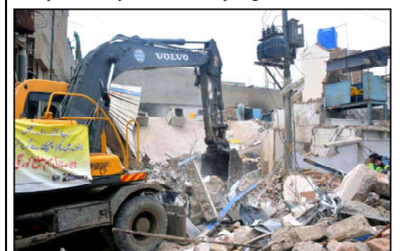
KARACHI: View of site after factory building roof collapse incident as rescue operation is underway, at Korangi PNT Society Gate in Karachi.
