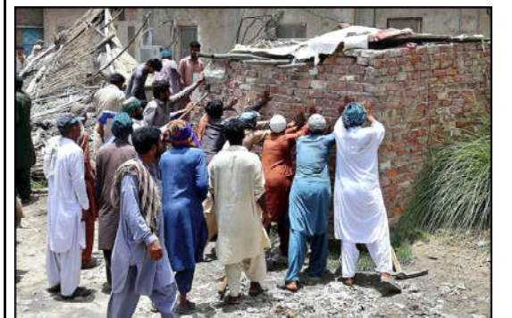
HYDERABAD: Railway staffers of Anti-Encroachment Cell demolishing encroachments at Makki Shah area.
