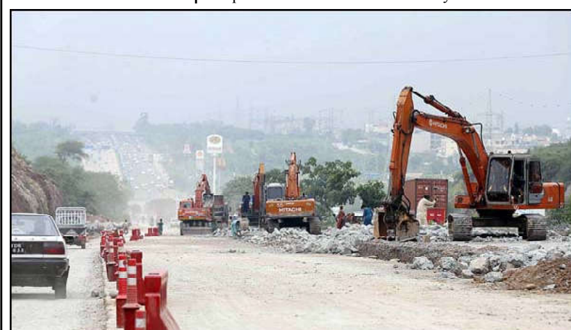
ISLAMABAD: Heavy machinery being used to build new lanes on Islamabad Expressway.
