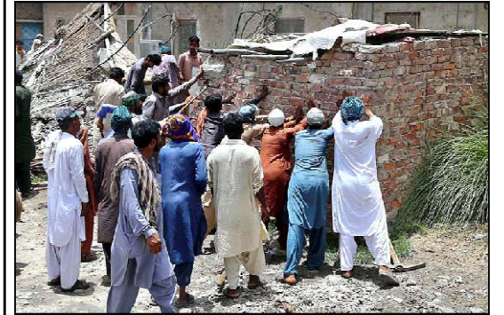
HYDERABAD: Railway staffers of Anti-Encroachment Cell demolishing encroachments at Makki Shah area.
