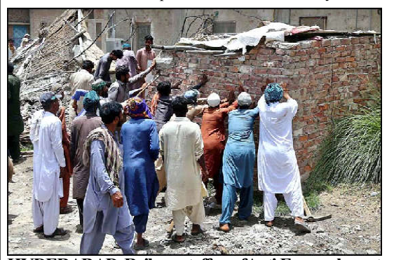
HYDERABAD: Railway staffers of Anti-Encroachment Cell demolishing encroachments at Makkhi Shah area.
