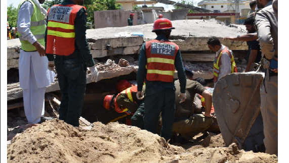
JHELUM: A view of site of gas cylinder explosion flattens three-storey building
