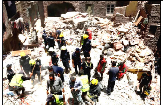
Rescuers search through the rubble of a collapsed five-story apartment building in Cairo, Egypt.
