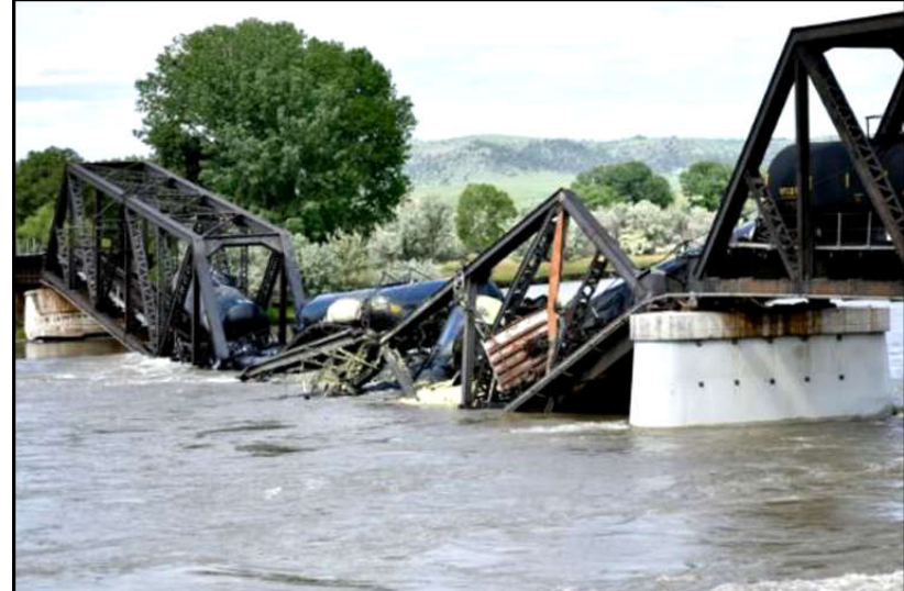
Several train cars are immersed in the Yellowstone River after a bridge collapse near Columbus, Mont.
