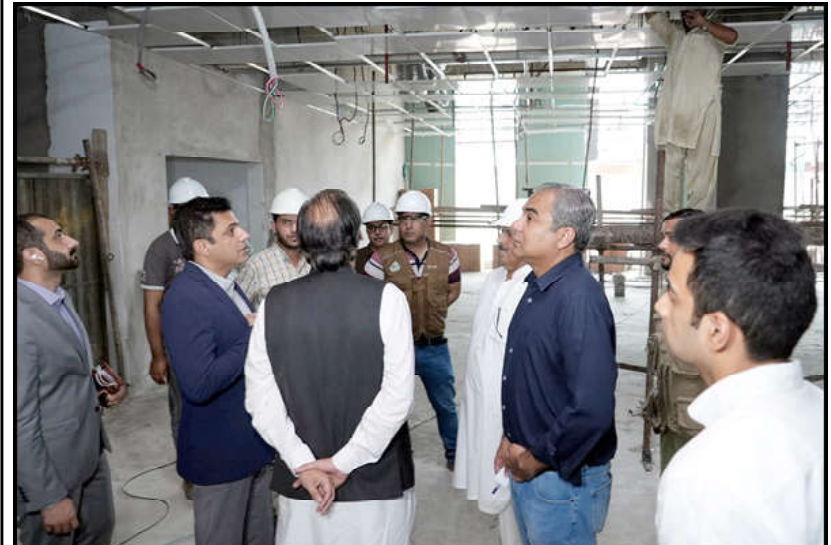
LAHORE: Caretaker Chief Minister Punjab Mohsin Naqvi inspecting the under construction work during his visit to Punjab Agriculture, Food and Drug Authority Project.
