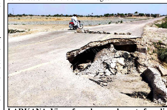
LARKANA: View of wreckage and worst of condition the bridge, needs the attention of concerned authorities, as its creating problems for commuters and they demand to concerned department to construction work as soon as possible, in Larkana
