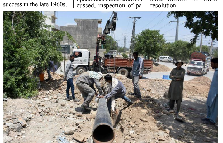
ISLAMABAD: Laborers are installing gas pipe line at Sector I-10 during high temperature, in Federal Capital.
