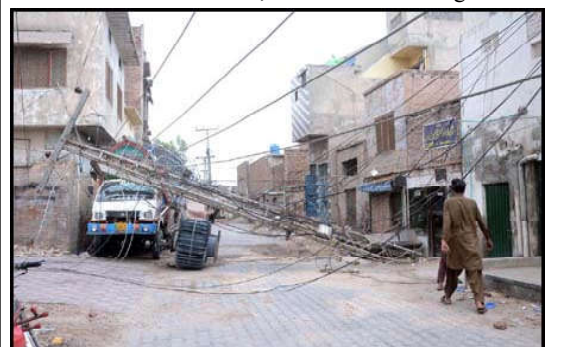
MULTAN: The unattended electric pole that fell two days ago at the Old Vegetable Market in Hassan Parwana Colony poses a potential accident hazard, demanding immediate attention from the relevant authorities.
