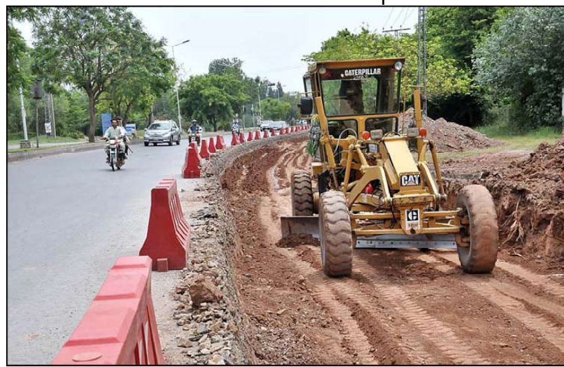
ISLAMABAD: Machinery being used for extension work of Park Road during development work in Federal Capital.
