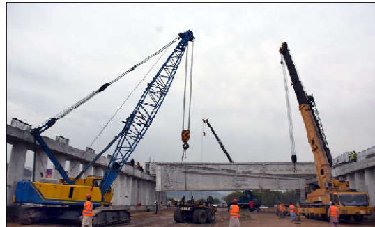
ISLAMABAD: Laborers are busy in their work during the construction of Fly Over at Sector E-11 as the 30th June is the final date of its Construction, in Federal Capital.
